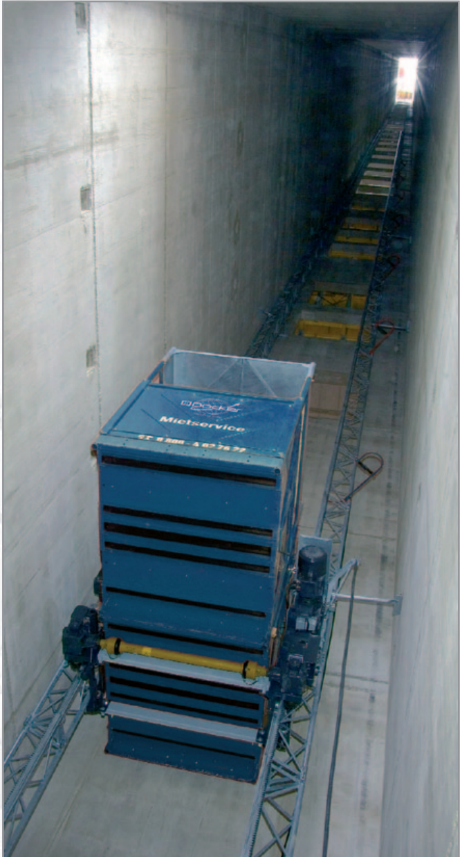
MX 1524-A34 installed in a lift shaft
